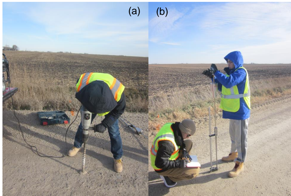
Figure 1. Dynamic cone penetrometer test: (a) drilling through macadam base layers and (b) performing the DCP test
