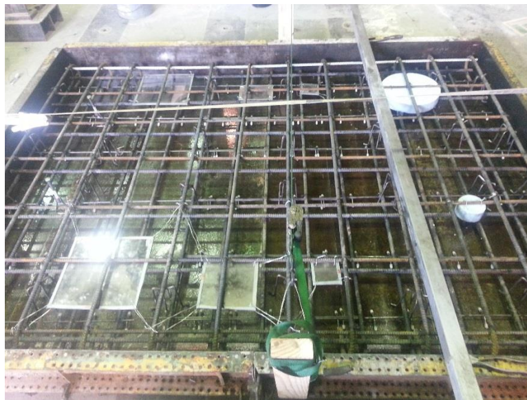
Figure 5.7. Formwork and rebar cage for mock-up bridge deck containing artificial defects before casting.
