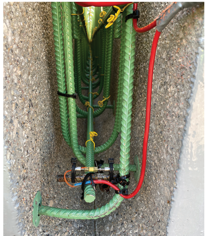
Embedded strain gauge at the bottom of a joint before concrete placement
