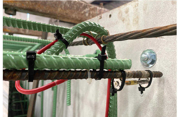
Embedded strain gauge at the top of a box girder before concrete pouring
